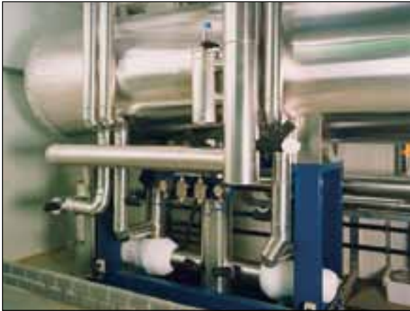
View of a CO 2 refrigeration plant with a pump system
